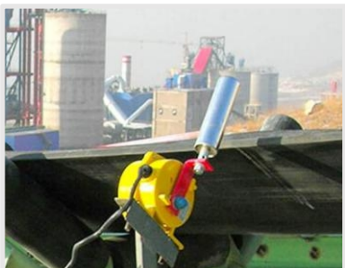
Belt Sway Switch
